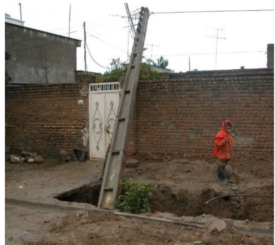
Figure 3. Subsidence of lamppost due to presence of collapsible soil in Gonbad-e-Kavoos
